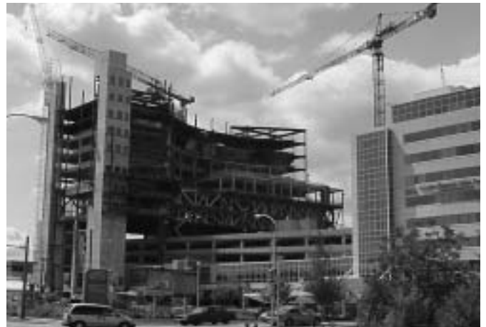
Boldt Construction officials say they improved jobsite production and achieved other benefits by applying lean principles to construction of this $182 million Cardiac Center project for St. Lukes Medical Center in Milwaukee Wis.
